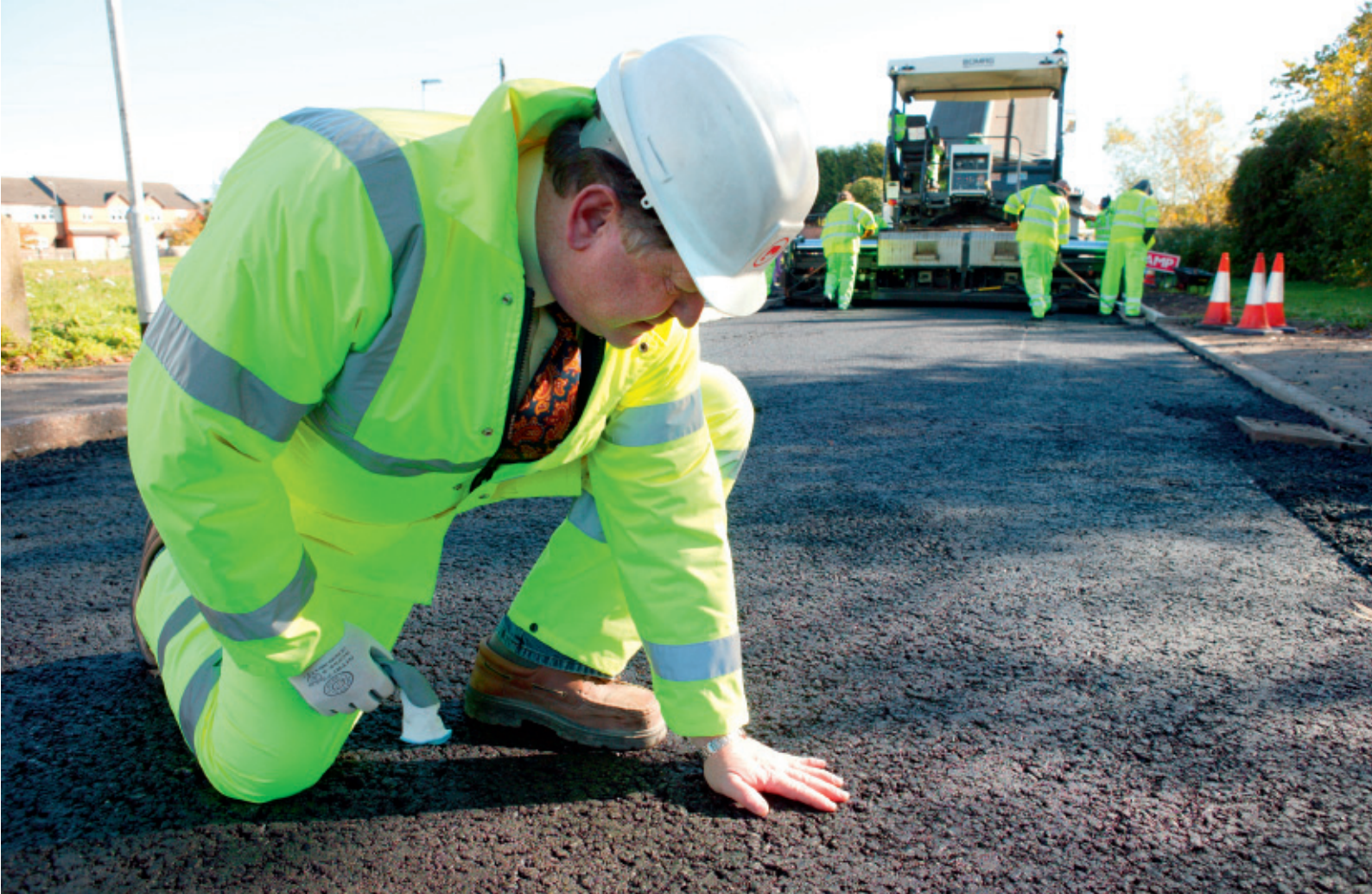
A Staffordshire pilot of the Low Energy Asphalt process proved a success. Over 7500t of the material has been supplied in the county this year
